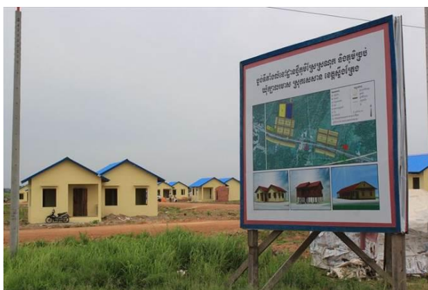
Unfinished resettlement site for Kbal Romeas communities along National Road No.78 (Photo taken on 25 th July, 2015)
