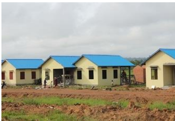
Unfinished houses at the resettlement site (Photo taken by a villager on 27 th July 2015)
