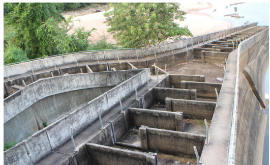
Fish Ladder at the Pak Mun Dam
